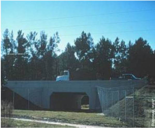
Figure 5.15: Fenced underpass for large wildlife (Defenders of Wildlife)
