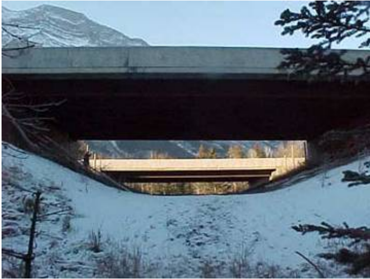
Figure 5.25: Wildlife underpass in Banff National Park, Canada (Clevenger, 2004)
