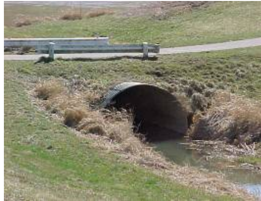
Figure 5.42: Culvert with standing water.
